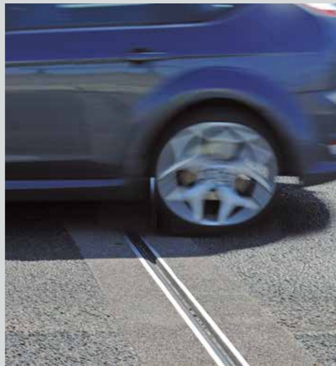
A close up of the BEJ expansion joint system not normally seen by the travelling public.
